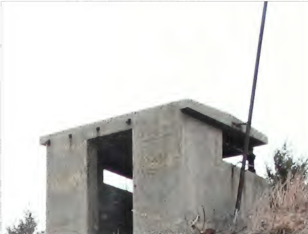
Figure 5.41. View of northwest facade of Battery Peck's commander station. The metal antenna and mounting brackets are features of this structure and should be preserved or replaced in kind. Measured drawings should be prepared to document these features followed by corrosion treatment, priming, and painting to match the historic finish (Olmsted Center, January 2009).
